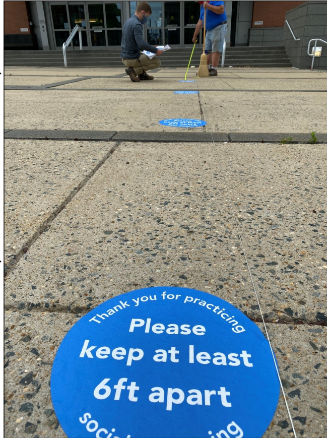
Work crews installing social distancing stickers outside the Leonard L. Williams Justice Center in July 2020.
