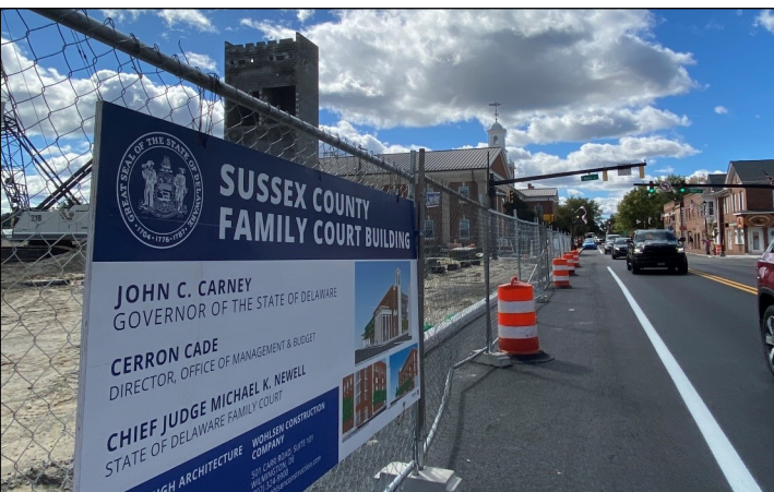
Construction at the site of the new Sussex County Family Court building in Georgetown, November/December 2023.
